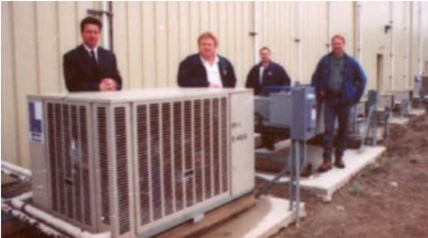
Pictured left to right: Duff O'Donnell, owner of EuroUSA, Dean Betlee of Controlled Environmental Systems, Jon Dresser of Refrigeration Sales Inc. and Paul Clement of Controlled Environmental Systems stand near a Larkin unit outside EuroUSA's warehouse.
