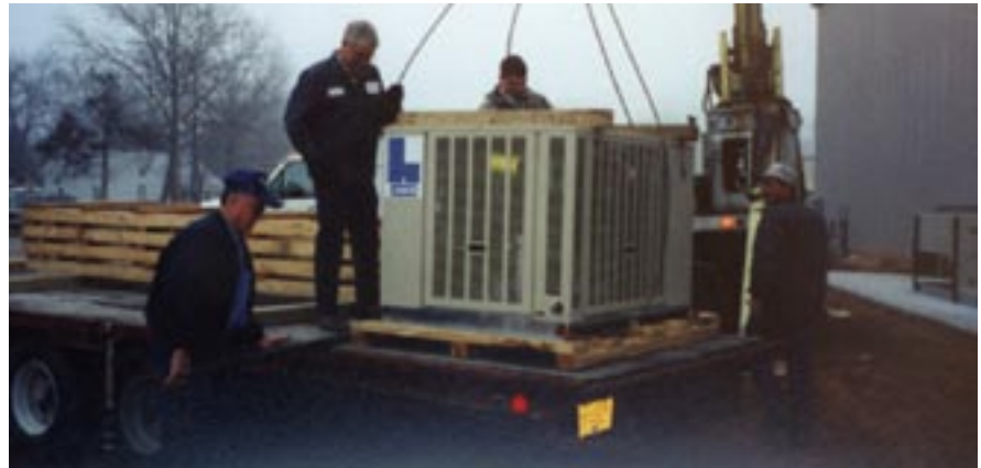
(Pictured left to right): James Neely, Patrick McAlister and Rick McAlister of Neely & McAlister, and Clint Granderson of Central Crane Services, prepare to transfer and install a Larkin condensing unit.
