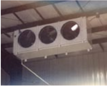
Larkin evaporators are used in the main storage area at M&K Distributors to cool cans, bottles, cases and kegs of Anheuser-Busch beer.
